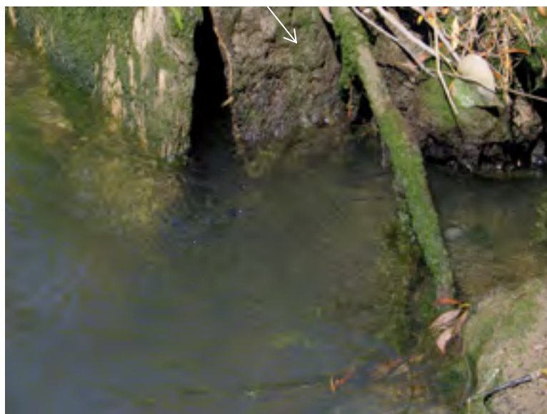
Figure 3. Motueka tide gate remains open even at half tide height, allowing about four to six hours on every tide cycle for whitebait to negotiate the culvert.
