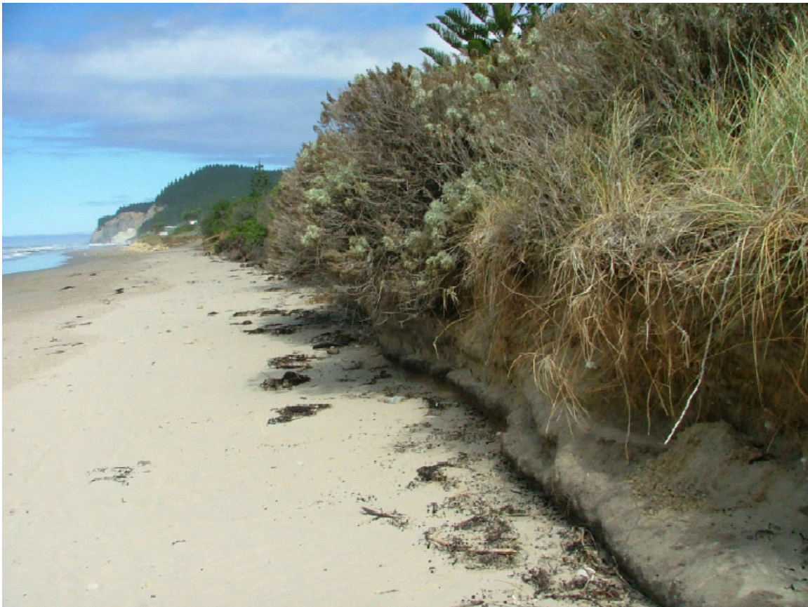
Figure 2. Foreshore erosion at Waimarama Beach (photo supplied by HBRC).
