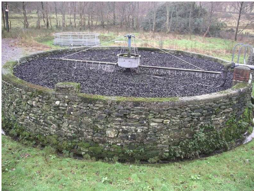
Figure 1 Trickling filter bed using plastic media for secondary sewage treatment
