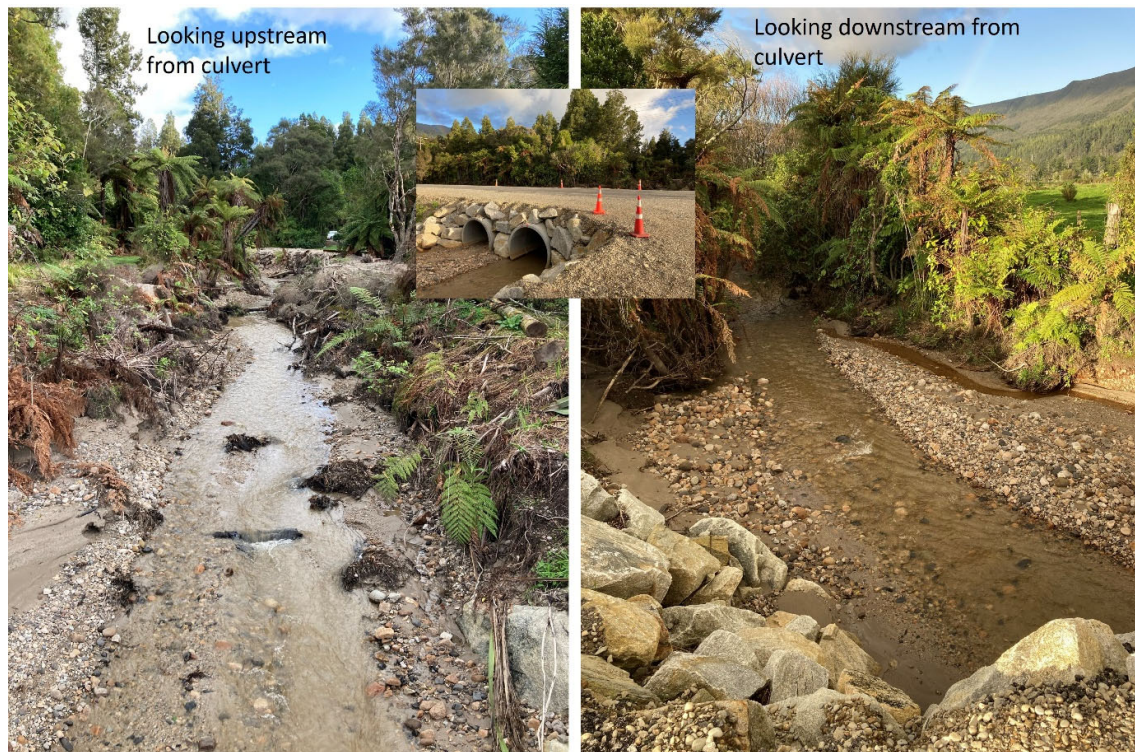
Figure 26. Lower Lake Stream channel (Crows Nest channel) in the vicinity of SH 67. Inset shows SH 67 culvert. 11 May 2022 (ICF).
