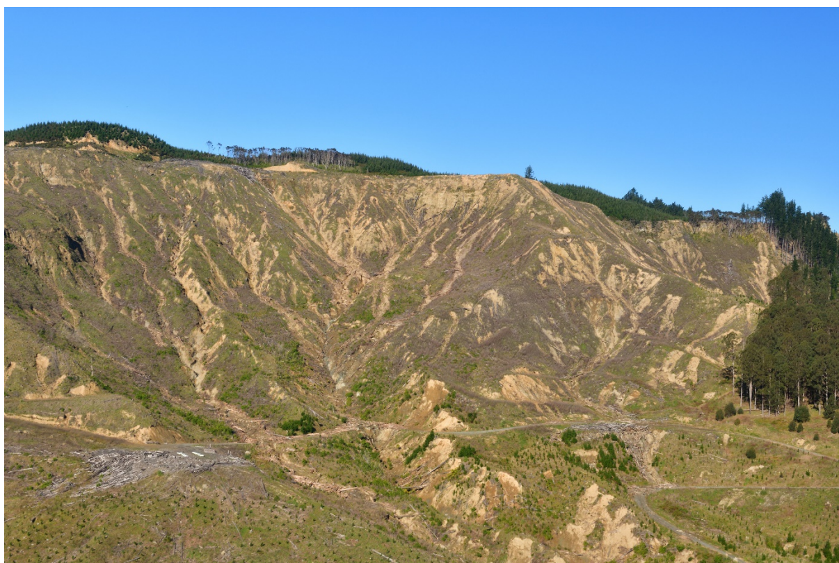
Figure 4.2 Extensive shallow soil slides, debris slides and debris flows in a newly forested area in the Mangatoitoi stream tributary of the Mangaheia River (Uawa Forest) (D. Townsend, GNS Science; 11 July 2018; D85_8017).
