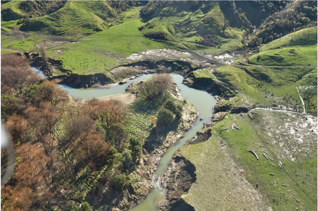
Figure 4.15 Bank erosion in the middle reaches of the Mangaheia River, downstream of Takapau Road/Wigan Bridge (D. Townsend, GNS Science; 11 July 2018; D85_7970).
