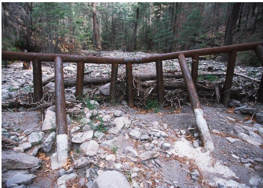
Figure 25: A substantial debris catcher ('Slash Rack') installed in a higher risk catchment (Photo retrieved from USDA NRCS)
