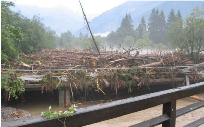
Figure 3: Mobilisation of woody debris is a worldwide problem; photo from Germany showing large-scale mobilisation by flood flow of whole trees from a catchment exposed to a major storm.
