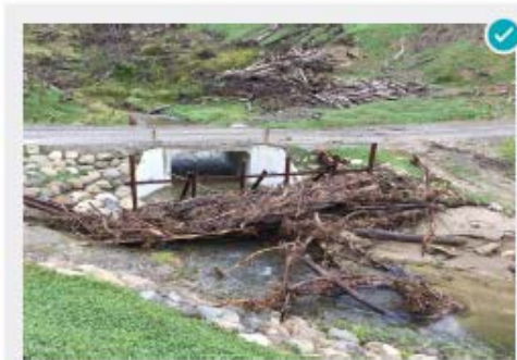
Slash captured by slash trap installed upstream of road and bridge. Accessible site allows removal of slash and maintenance of the slash trap.
