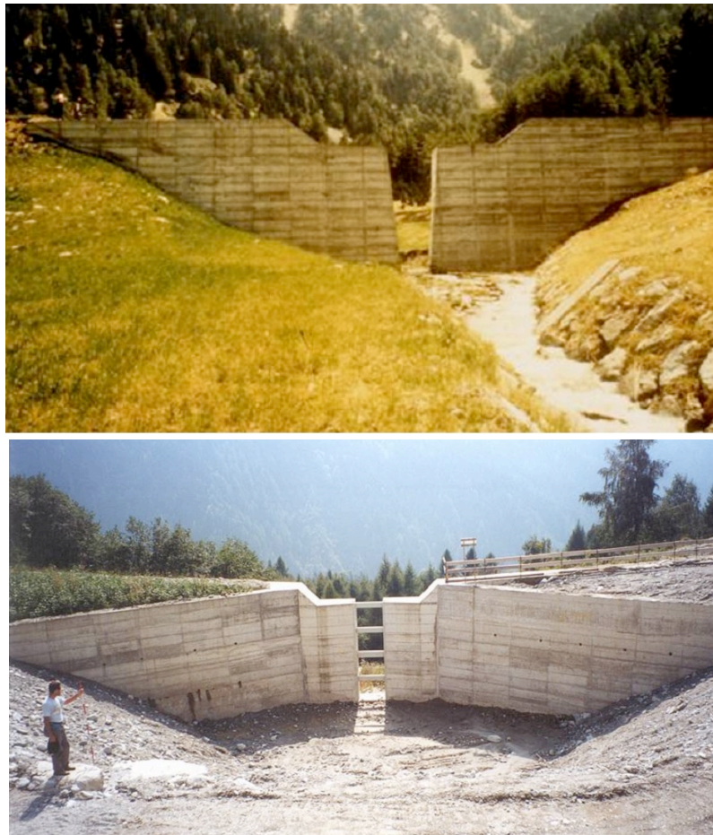
Figure 8: Photos of two similar designs, whereby the lower structure design to retain more woody debris with horizontal elements to restrict passage of larger and medium-sized woody material,
