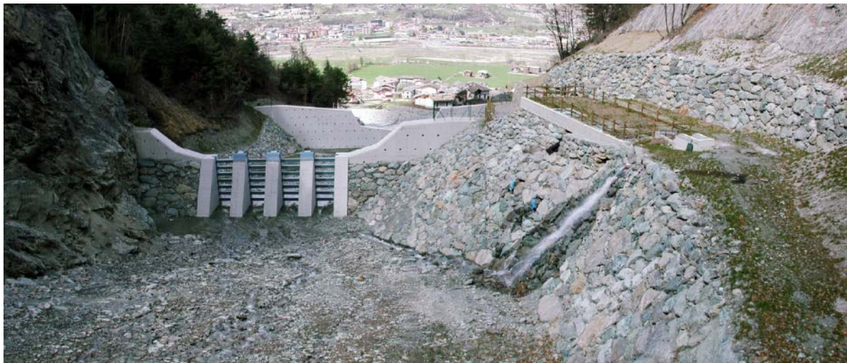
Figure 17: Substantial modification of the natural waterway to prevent debris from impacting communities downstream. Design elements include a series of dams, including the slash-catching component in the first structure, as well as embankments to prevent scour.
