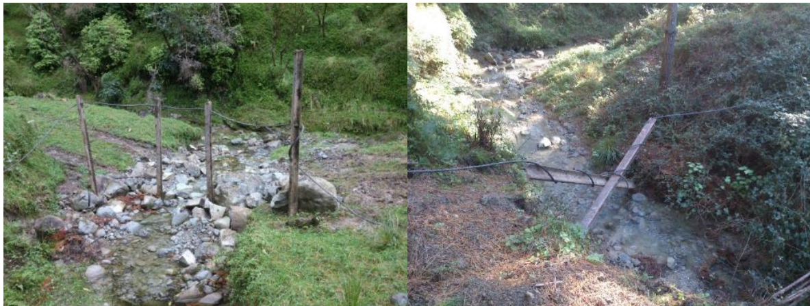
Figure 24: Left - Slash trap in a headwater stream using crossed railway irons embedded in the stream bed. Wire rope is wrapped around the railway irons and secured. Right - slash trap installed using vertical railway irons with wire rope is threaded through the irons and secured either to mature trees or to deadmen anchors (buried logs).
