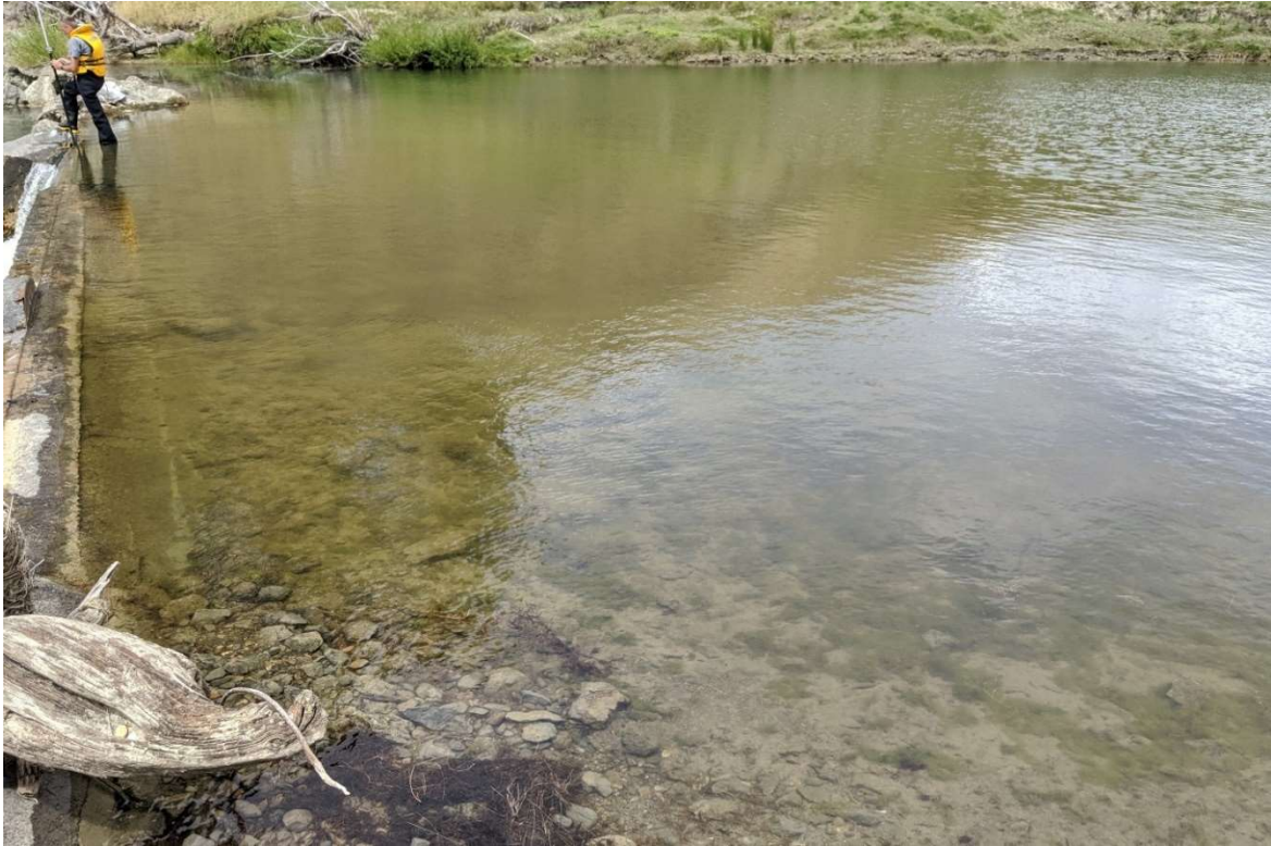
Figure 3-7: The lower weir viewed from upstream. Note the infilling of sediment behind the weir.
