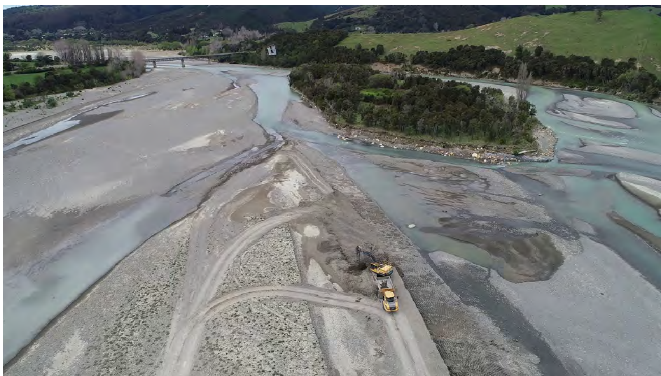
Figure 2-4 Extraction works near the Rotokautuku Bridge (SH35) are carried out using a combination of skimming the bar surface, as well as deeper elongate trenches, parallel with the flow.
