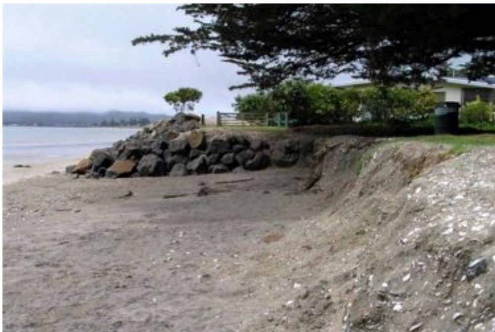
Figure 10-1: Erosion beside a sea wall in Whitianga. Photo: R. Bell, NIWA.
