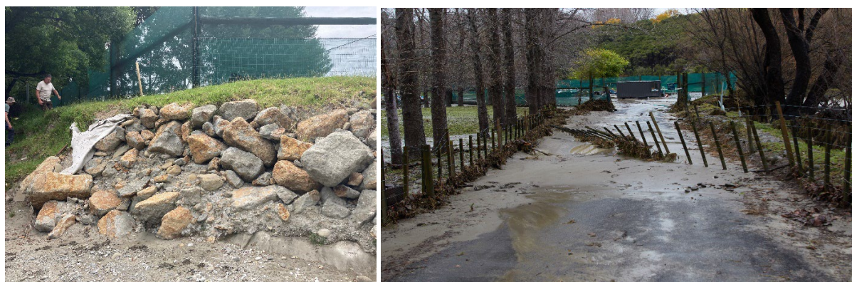
Figure 19. Left: damage to rock revetment protecting landfill site, photo: 30 November 2021 (ICF); right: washover of approach road to landfill site, photo: 20 June 2021 (Murry Cave).
