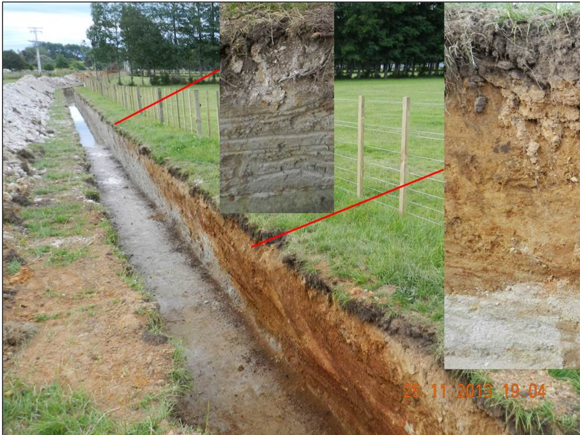
Figure 25. Excavation for a buried power cable reveals the transition from a redox mottled Brown Soil (foreground) to a Gley Soil. Note the summertime water table in the distance and the grey colours mid-photo indicating the extent of the winter time water table. An iron pan was present in the transition zone between Brown and Gley Soils.
