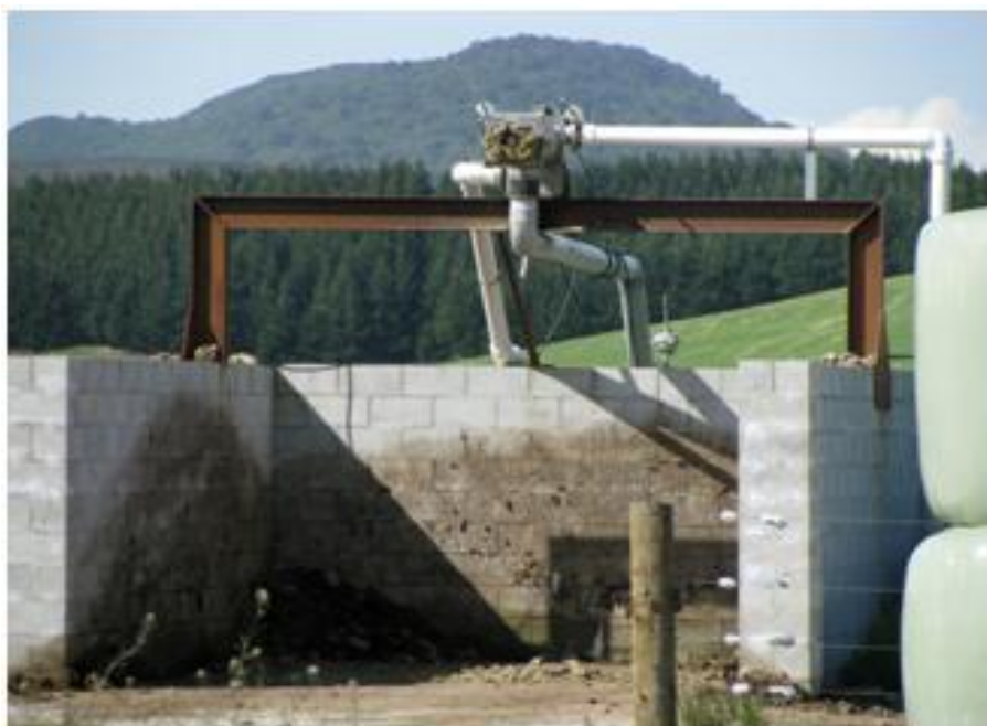
Photo 38: Screw press solids separator on raised platform above solids bunker.
