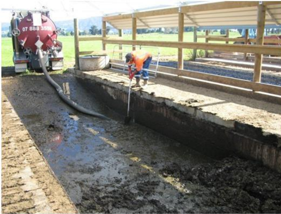
Photo 9: Liquid sucked out of manure bunker before solids removed.
