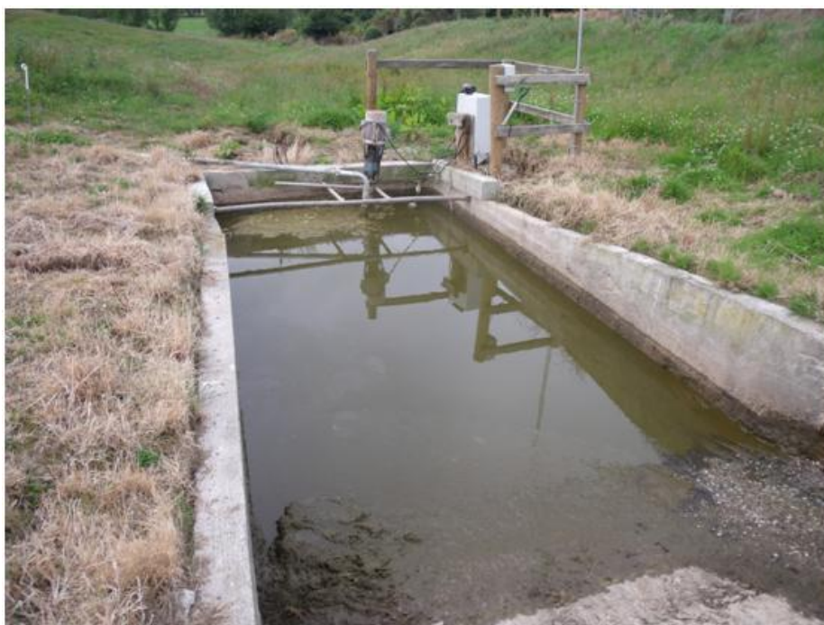
Photo 43: Sand/stone sump with raw FDE.
