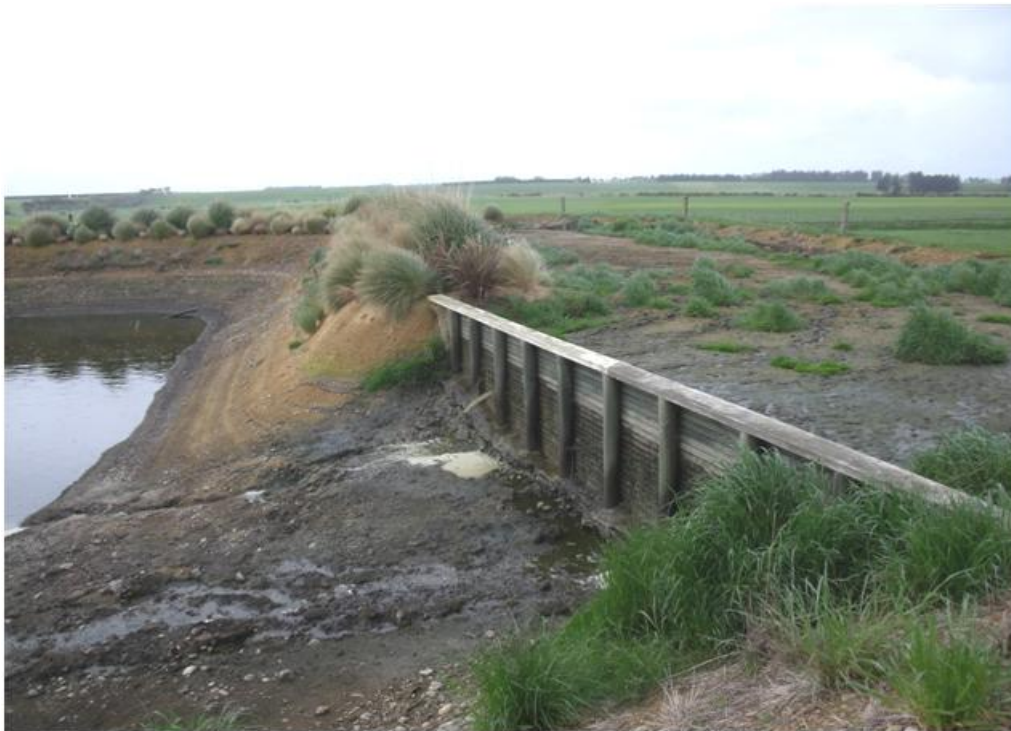
Photo 48: Weeping wall solids with liquid draining to effluent storage pond.
