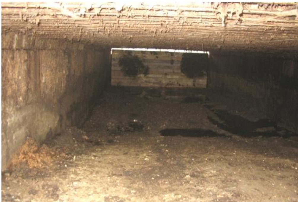
Photo 26: Weeping wall inserted near back of manure bay to drain off liquid.
